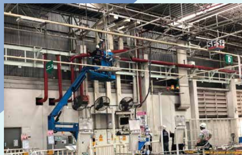
Fire Alarm System
