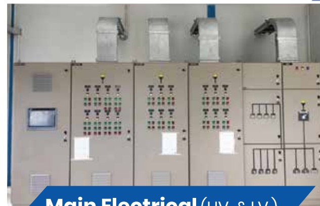
Main Electrical (HV. & LV.)
