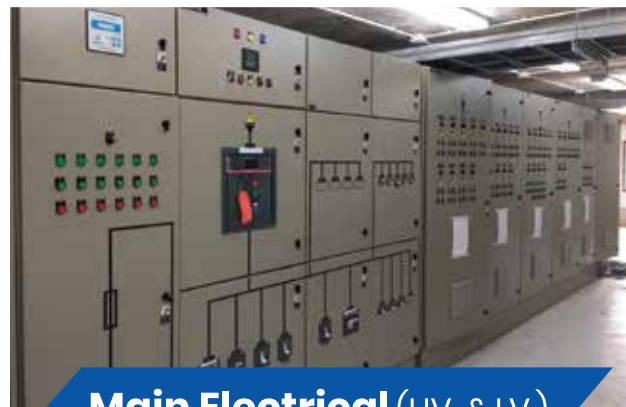
Main Electrical (HV. & LV.)
